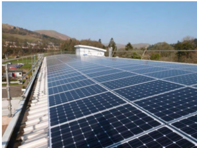
Solar panels at Langholm Academy
