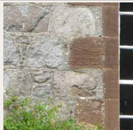
near Kelton; rubble wall with pinning ( the use of smaller stones, or pinings, to "fix" larger stones into the wall ) and contrasting dressed surrounds at windows.
