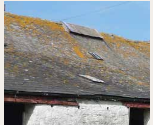
lichen on roof
