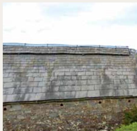
ventilators at ridge
